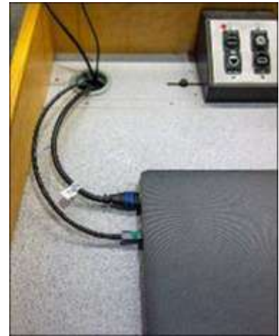
Classroom Laptop cable connections
