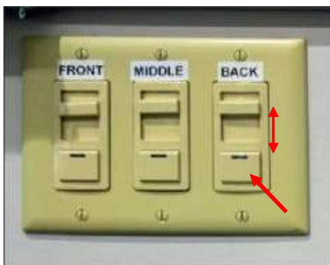
Ceiling Light Bank Switches (on/off & dimming slider)
